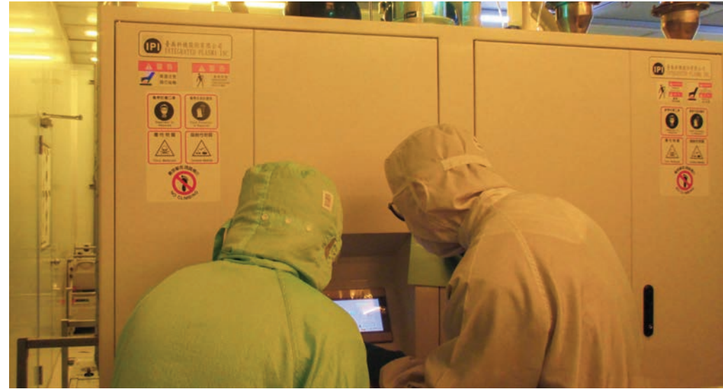
Amkor Taiwan team operating F-gas abatement system.
