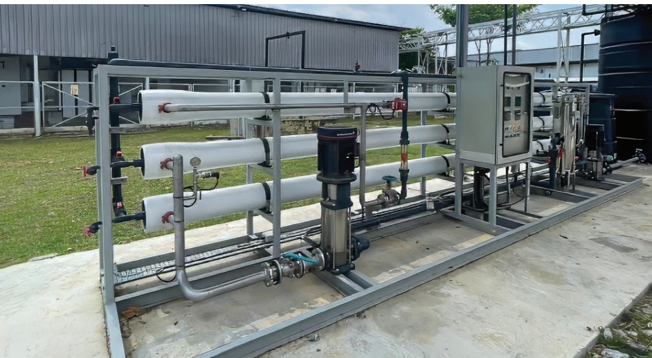
RO system installed in Malaysia.
