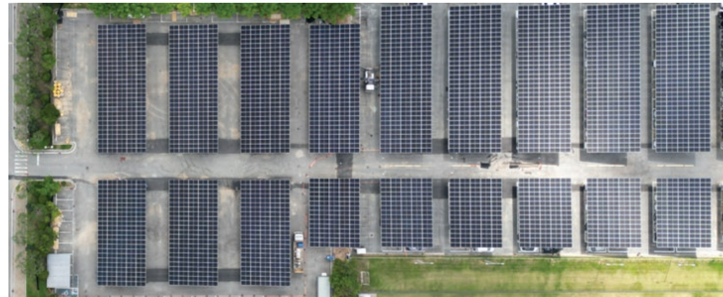
Solar PV system at our site in South Korea.
